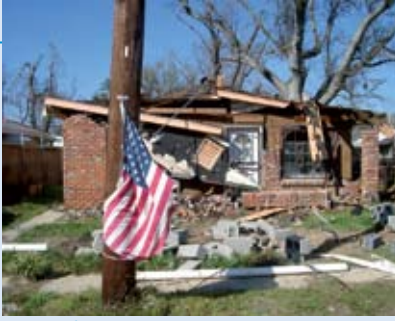
Damages from Hurricane Katrina, © Munich Re
